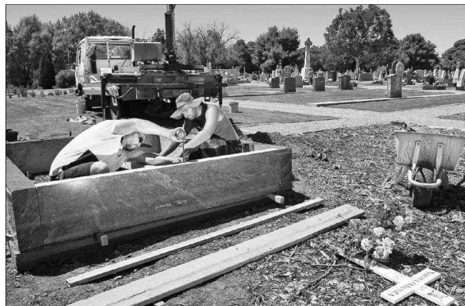
LABOUR OF LOVE: Sean and Andrew, from Italian Monumental Art, install a new structure at West Terrace Cemetery.
